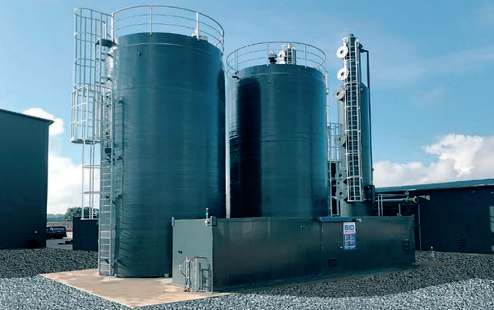
FIGURE 5.4 Biogascleaner QSR desulphurization plant at Nature Energy Maansson in Brande, Denmark. PHOTO Biogasclean.
