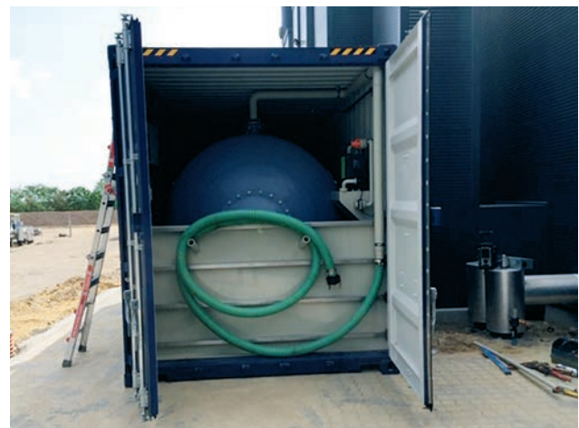
FIGURE 5.7 Storage tank installation as a container solution. PHOTO Kemira.
