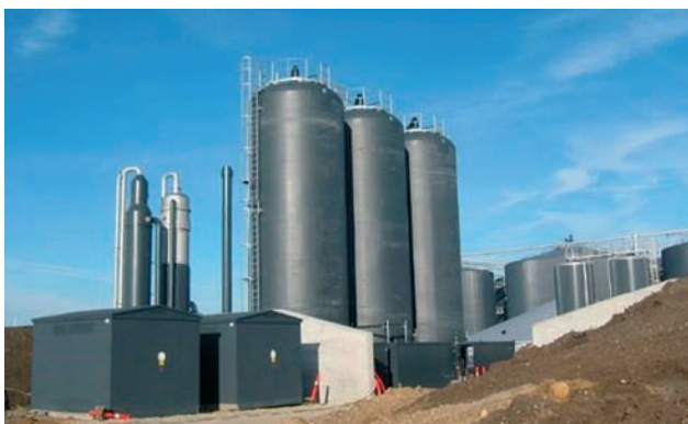
FIGURE 5.5 Biogascleaner QSR desulphurization plant to NGF Nature Energy Korskro in Denmark. PHOTO Biogasclean.
