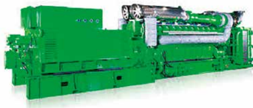
FIGURA 5.8 Gas engine and generator for biogas plants provided by Jenbacher. FOTO Jenbacher.
